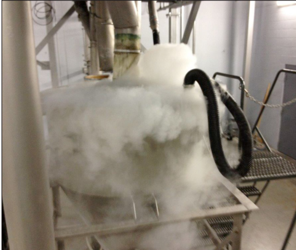
Conveying dry ice through the piping can remove build up and deposits in the line
