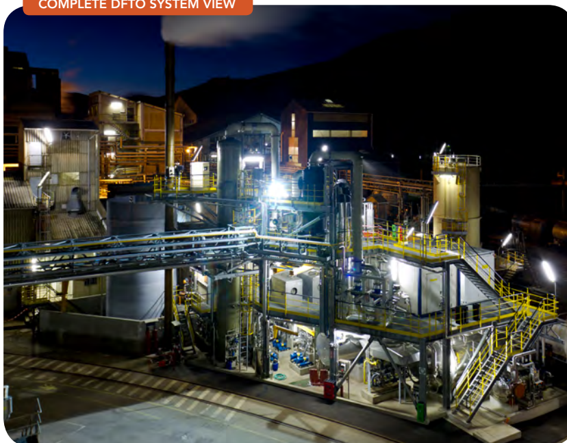
Figure 5. This DFTO system helped reduce fossil fuel use in boilers and eliminate offsite waste disposal costs.
