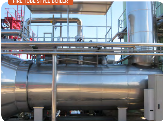
Figure 2. The system includes a fire tube, single pass waste heat boiler to generate medium pressure saturated steam.
