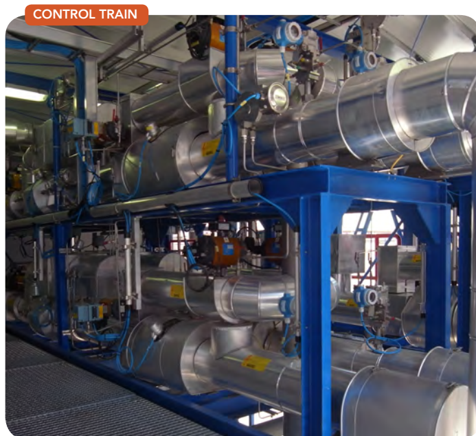
Figure 1. The thermal oxidizer system controls six process off gas streams, each handled by multiple skid-mounted off gas piping control trains.
