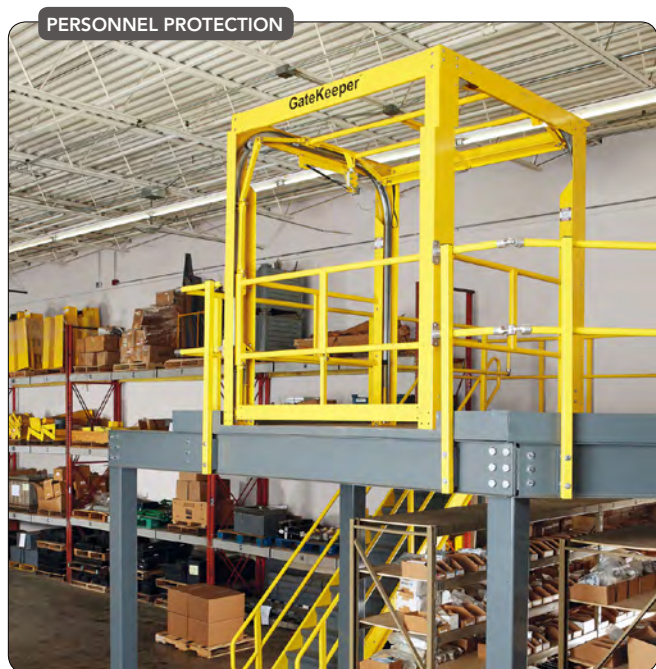
Figure 3. This dual reciprocating barrier makes elevated platform loading and unloading safer.
