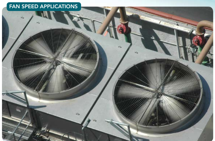
Figure 3. Using a reducing coupling and a variable frequency drive can simplify fan speed adjustments.
