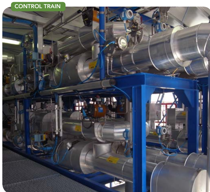
Figure 1. The thermal oxidizer system controls six process off gas streams, each handled by multiple skid-mounted off gas piping control trains.
