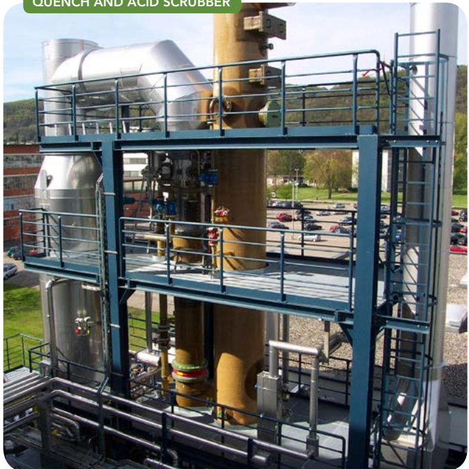
Figure 3. After exiting the economizer, the flue gas is directed to a quench and acid scrubber, much like this one.
