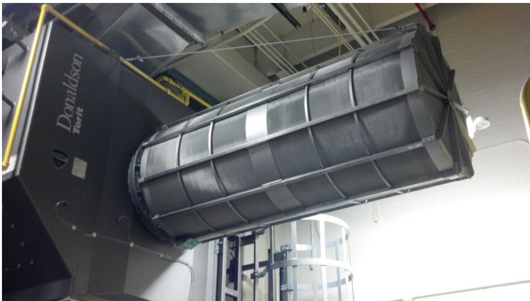
Figure 1. A flameless vent installed in a manufacturing facility is an economical and safe means of eliminating the risk of damage and fatality from dust explosions.
