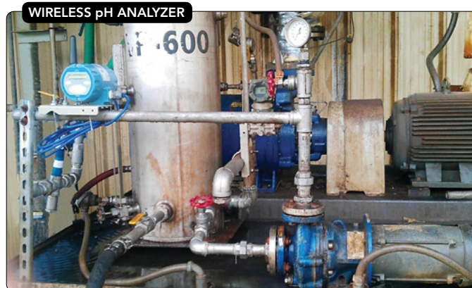
Figure 1. Unit monitors seal fluid to safeguard against corrosion of vacuum pump.
