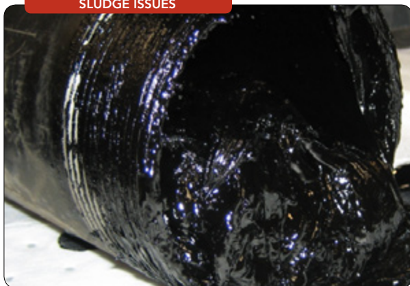
Figure 4. Sludge accumulation as a result of oxidation can cause low-flow zones, plugged lines and cold-spots.
