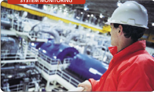
Figure 5. Periodic monitoring, including a walk through, of your thermal fluid system are essential to prolonging a safe and predictable system.
