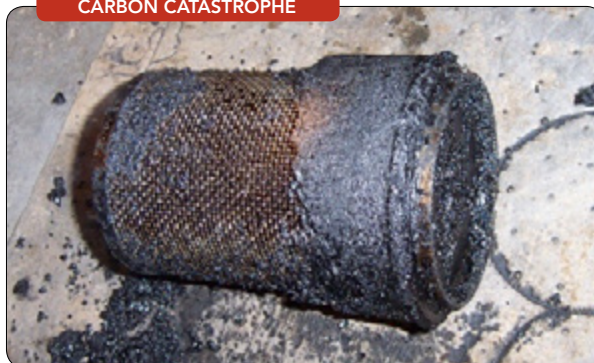
Figure 3. Severe carbon buildup in a strainer basket resulting from unmonitored thermal degradation.
