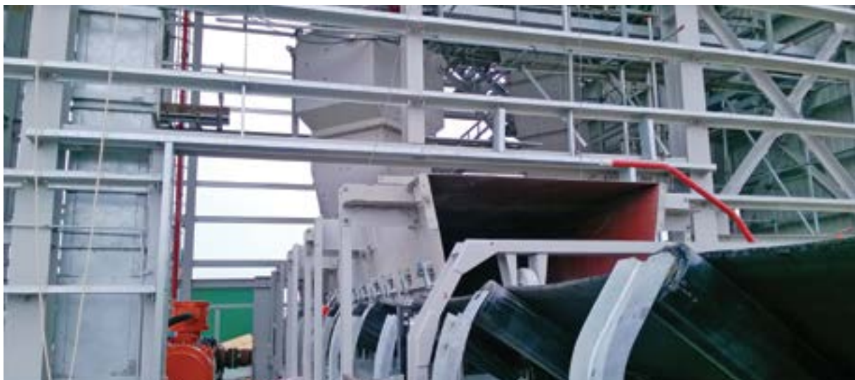
Figure 1. Skirting on belt conveyor at the loading/impact point (tail end) extends sufficiently to reduce dust propagation.
