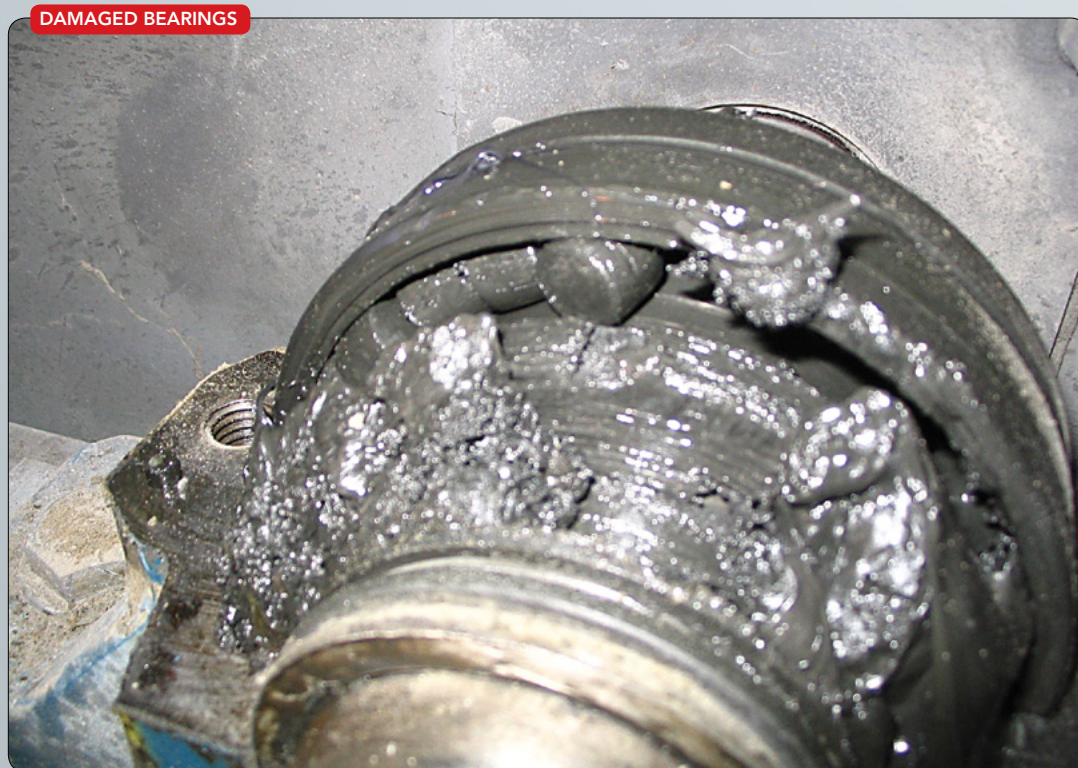
Figure 1. Missing or out-of-position roller bearings lead to telltale vibrations.
