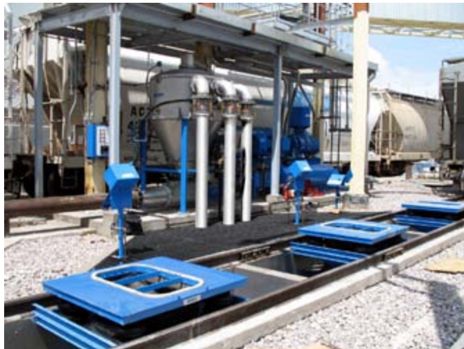
Figure 2. Three Cyclonaire CycloLift™ railcar connectors were installed beneath the tracks to streamline rail unloading from the hopper-bottom cars and eliminate spillage.
