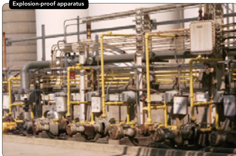
Figure 2. Checking the tightness of lids and terminals and for corrosion and deformation is essential.
