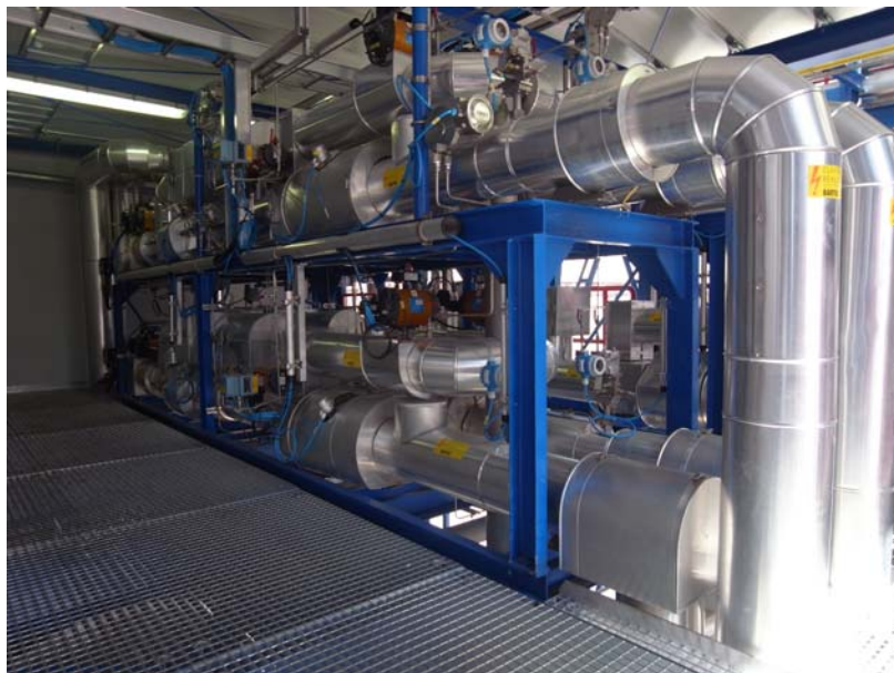
Multiple skid-mounted off gas piping control trains
