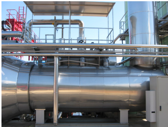
Fire tube style, single pass waste heat boiler
