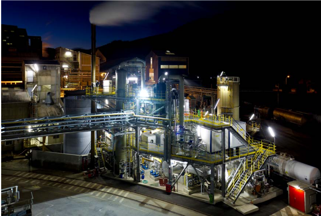
Complete DFTO system view
