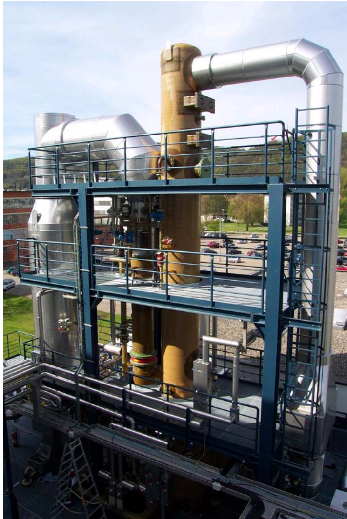
Typical quench and acid scrubber after a DFTO
