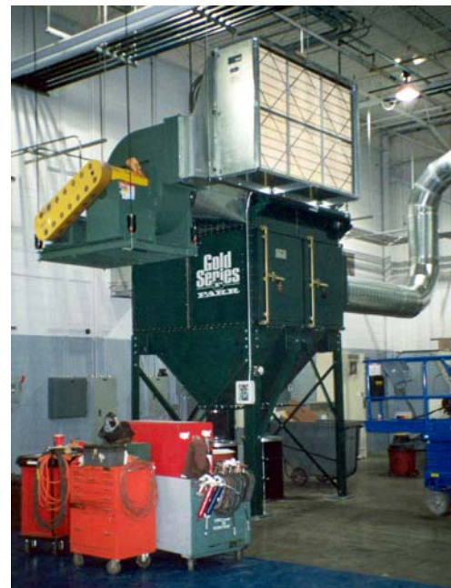
Dust collector installation on a plastic powder mixing application.
