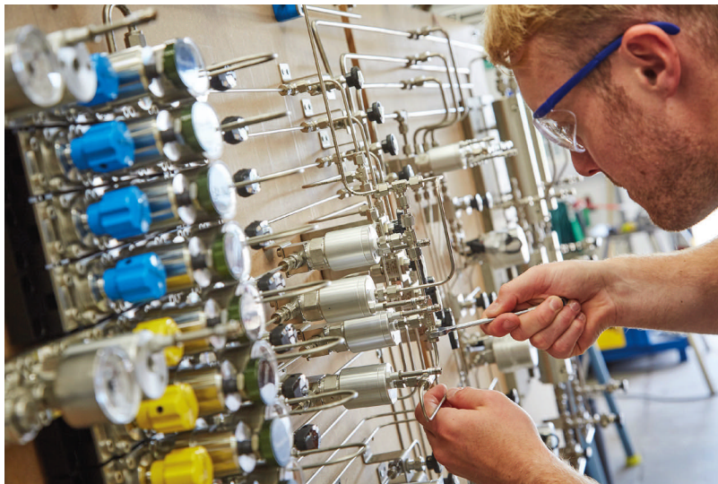
Figure 1. Newer gas pressure control panels are often designed in ways that are more intuitive for maintenance technicians, decreasing the time, labor, and costs associated with keeping them in working order compared to legacy systems. Images © 2023 Swagelok Company
