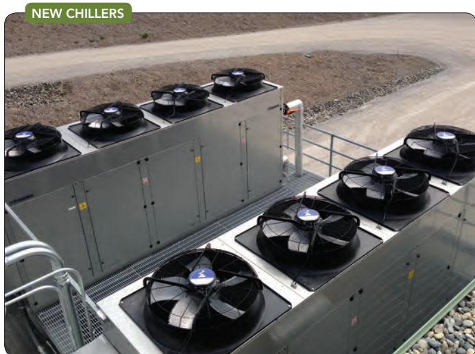
Figure 1. Two R1270 units, each with 260-kW cooling capacity, chill brine at a plant in Orlando. Source: Versatile Refrigeration Inc.
