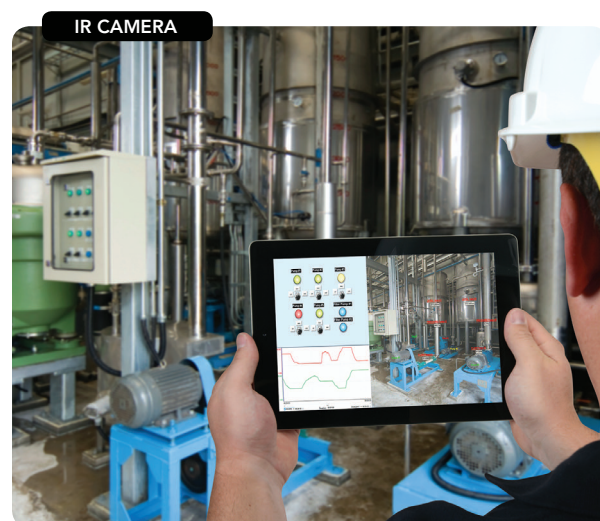
Figure 2. Readings from a camera can provide the first warning of a leak, and spur follow-up checks with a flame ionization detector. Source: Sage Environmental.
