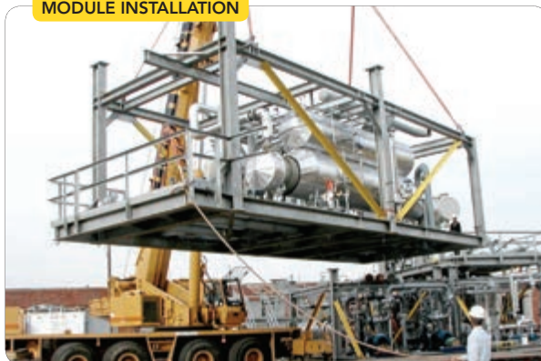
Figure 2. Fabrication in a shop instead of in the field usually provides equipment faster and at lower cost. Photo courtesy of EPIC Process Systems.
