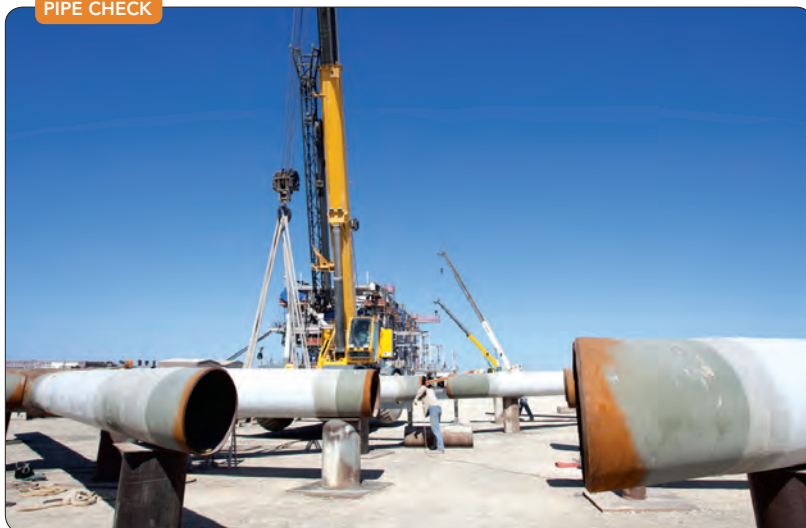
Figure 3. On new builds, it is essential to confirm that protective coatings are applied properly and the underlying metal meets spec. Source: AkzoNobel.
