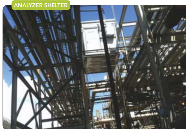
Figure 1. Analyzers usually must reside close to the monitored operation — and this dictates the shelter site.
