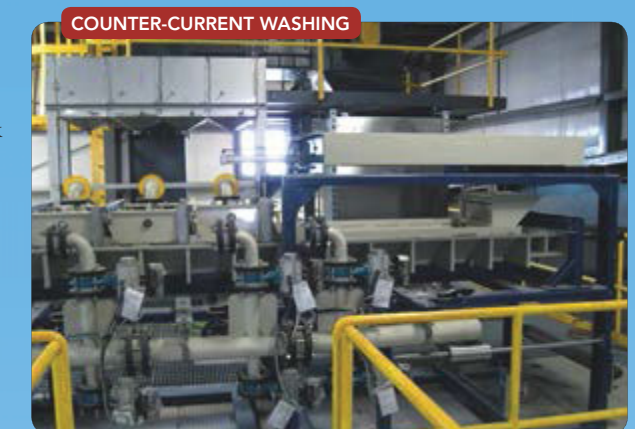
Figure 1. Boxes on top of structure feed wash devices on belt filter. Source: BHS-Sonthofen.
