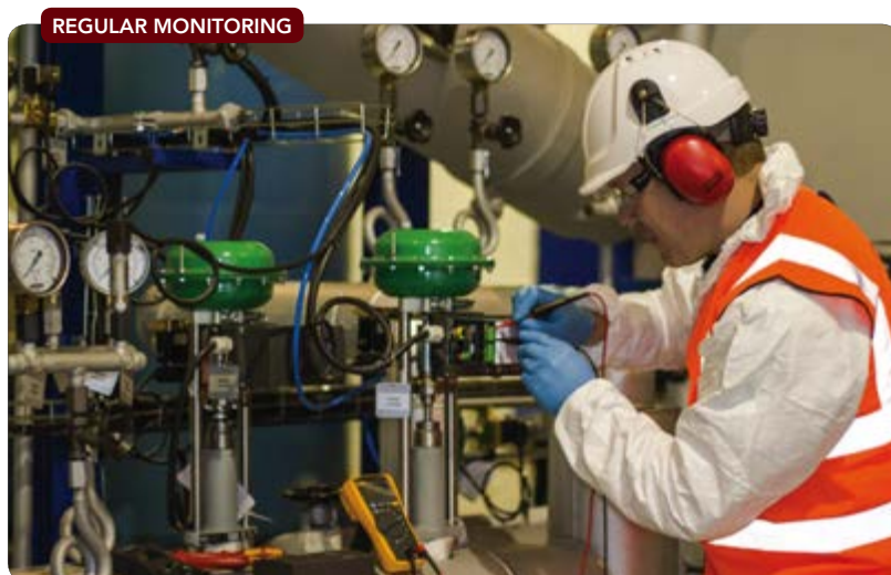
Figure 1. Maintaining optimum performance requires effective ongoing maintenance.
