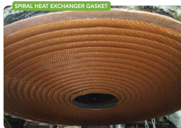
Figure 2. Disassembly after more than six months' service revealed gasket was still in good condition.
