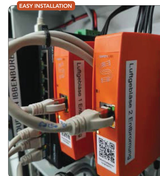
Figure 1. Sensor mounts in electrical cabinet rather than on rotating equipment. Source: Nouryon Industrial Chemicals.
