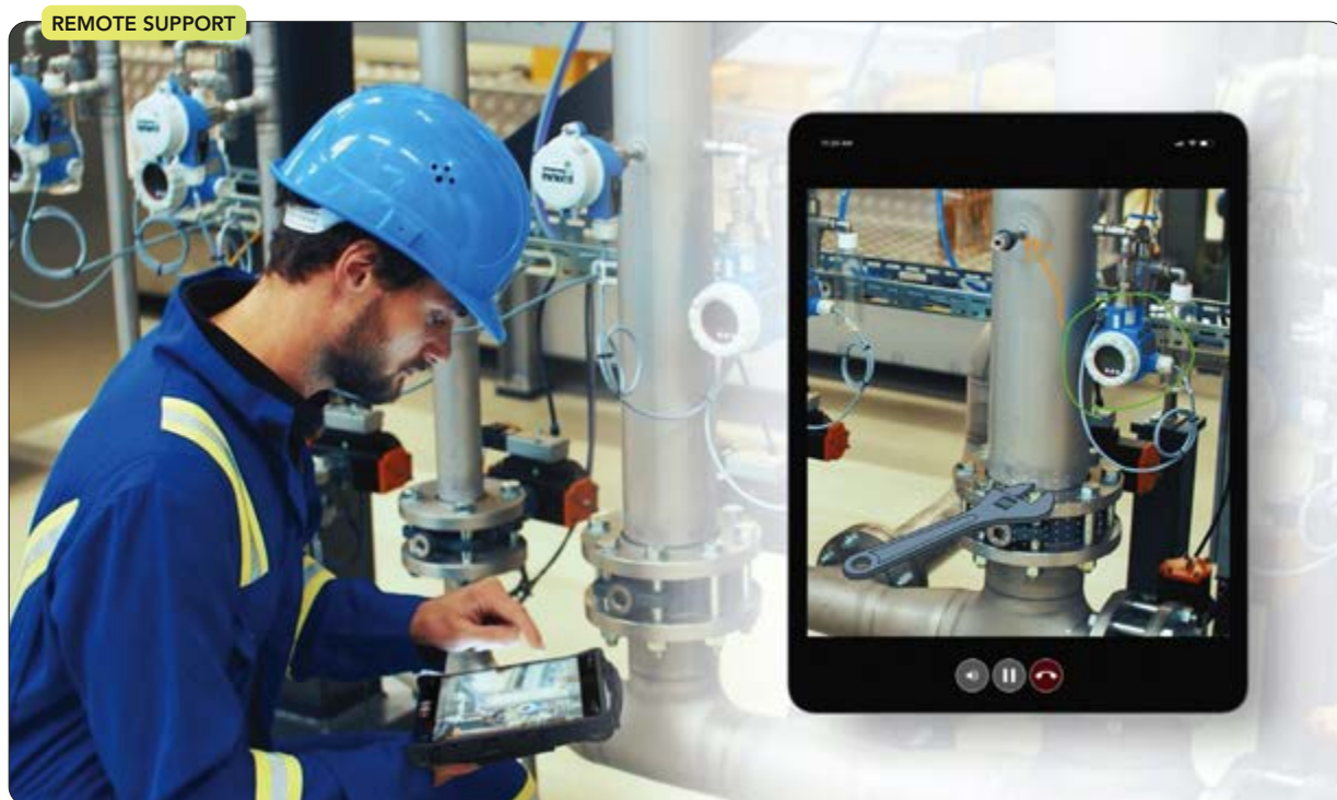
Figure 2. Off-site experts use live video streams to help plant personnel deal with instrumentation issues. Source: Endress+Hauser.
