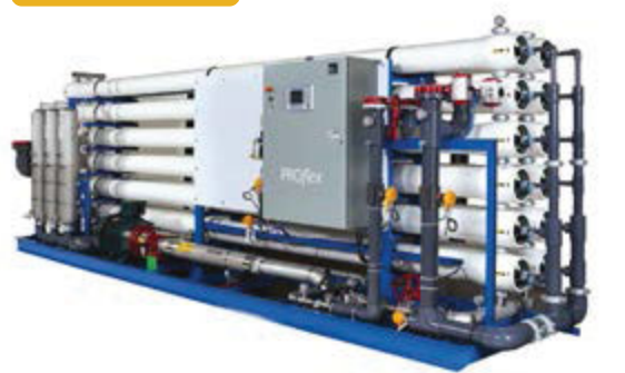
Figure 1 Membrane systems such as PROflex can concentrate organic contaminants in a waste stream. Source: Suez Water Technologies & Solutions.
