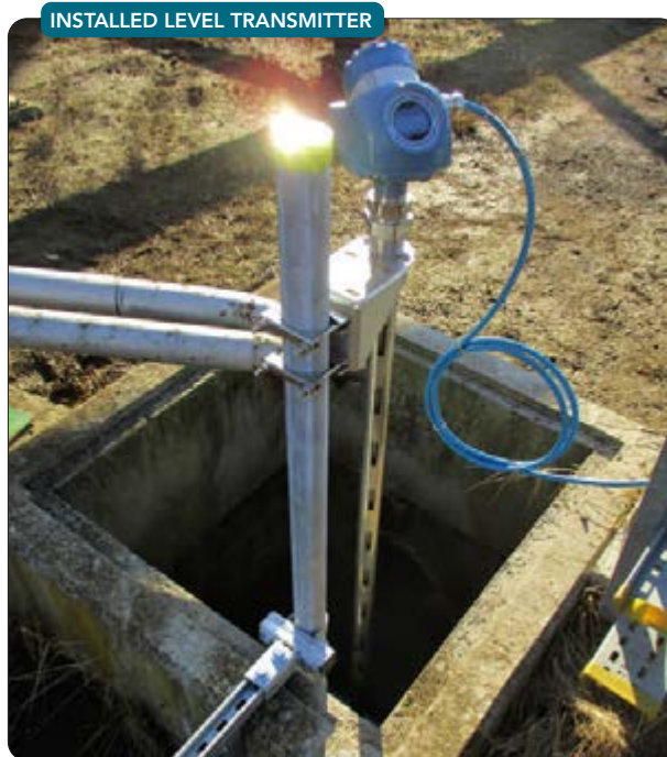
Figure 3. Site is using 44 of these transmitters for automated monitoring of secondary containment areas to provide greater visibility of potential leaks.
