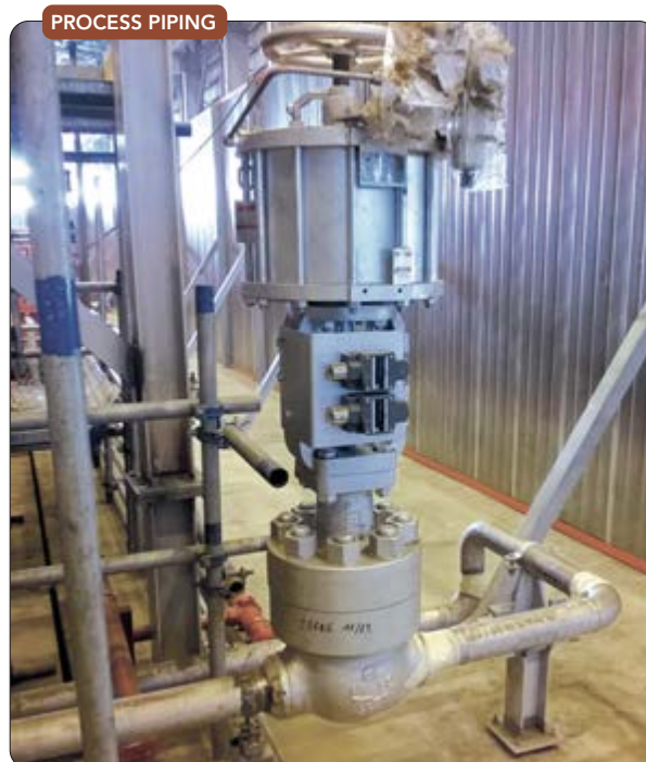
Figure 1. This piping, shown during construction, requires careful stress analysis to ensure it can cope with attached equipment.
