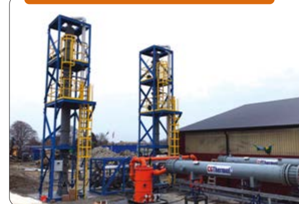
Designed to condense HCl entrained vapor for a soil remediation project in Sweden.
