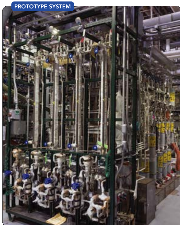
Figure 1. Pilot unit in New Jersey contained four reactor trains and had about 130 I/O points.
