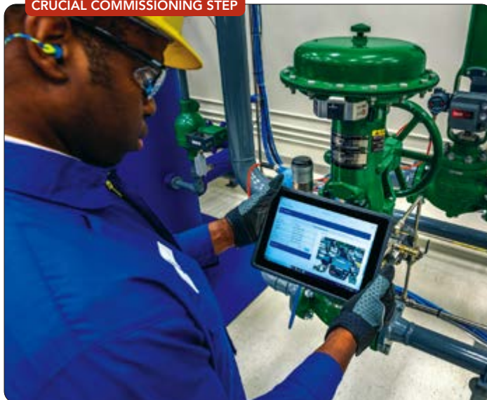
Figure 5. Capturing a post-repair stroke signature provides critical data for spotting developing problems.
